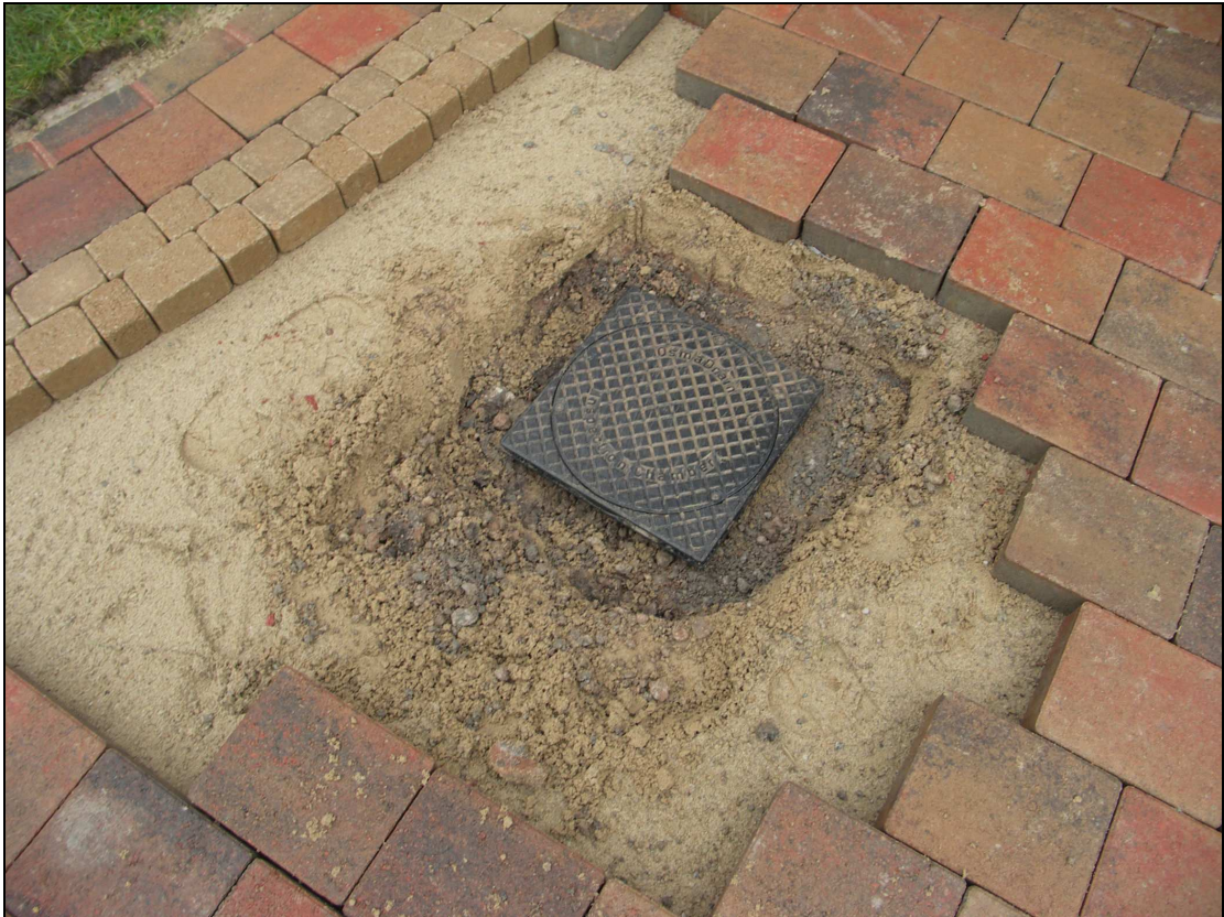
Figure 1 - AC 1 - Old cover in place
